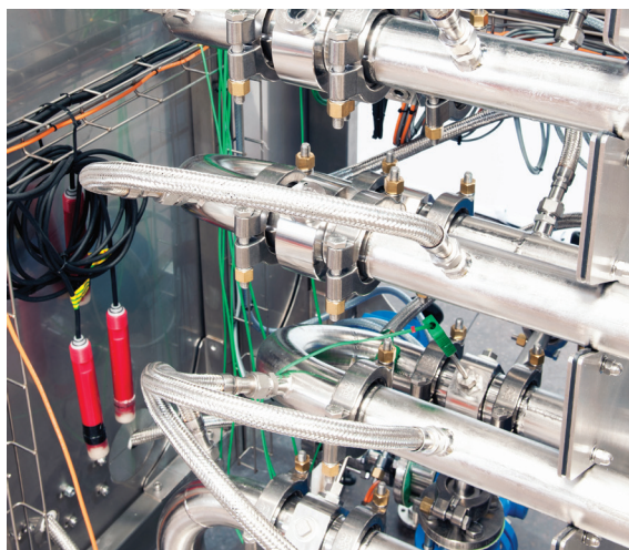
A Croda unit for making an emulsion in a UK company
